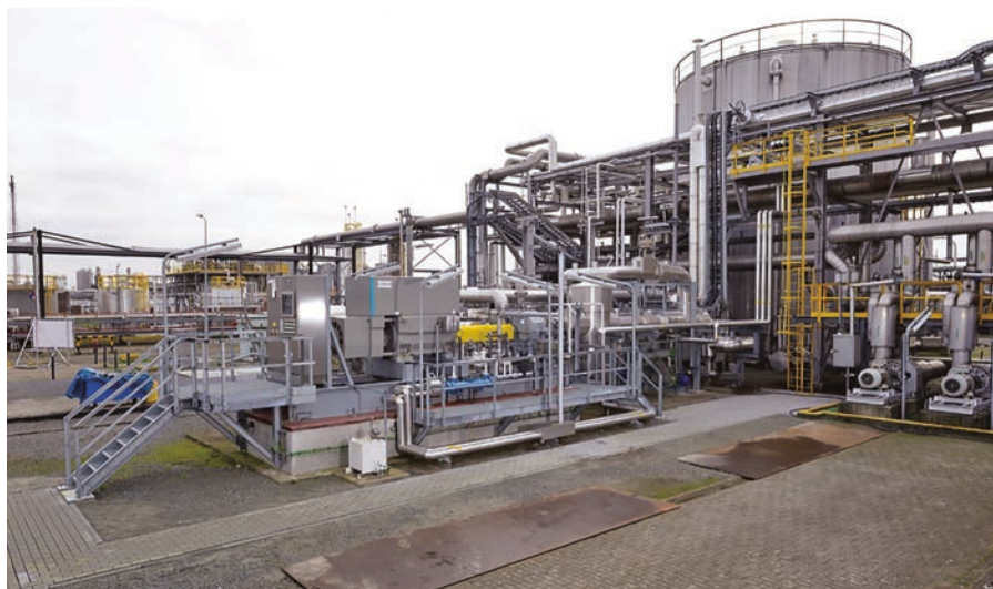
FIG. 4. The compressor installation inside the Terneuzen plant.
