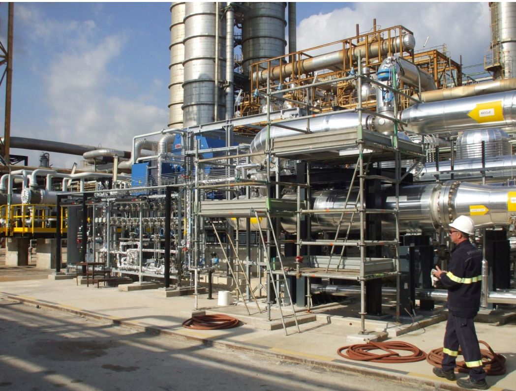
MVR for a petrochemical plant in Sicily, Italy (source: Atlas Copco)
