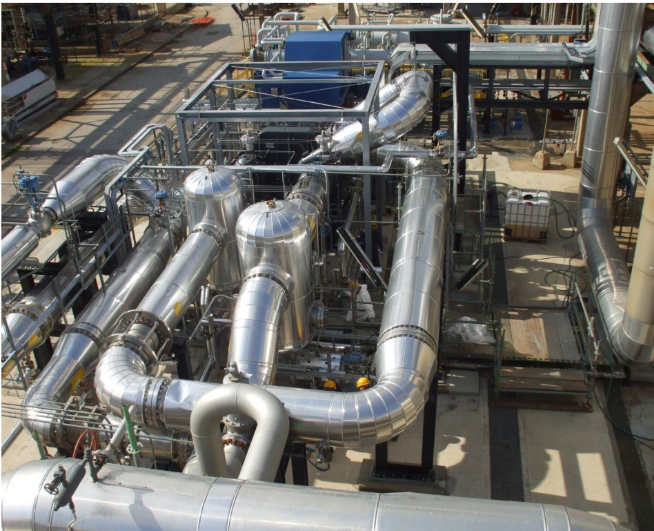
MVR for a petrochemical plant in Sicily, Italy (source: Atlas Copco)
